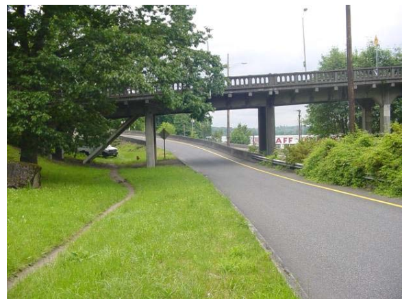
Figure 8: Worn pedestrian path along west side of southbound loop ramp.
