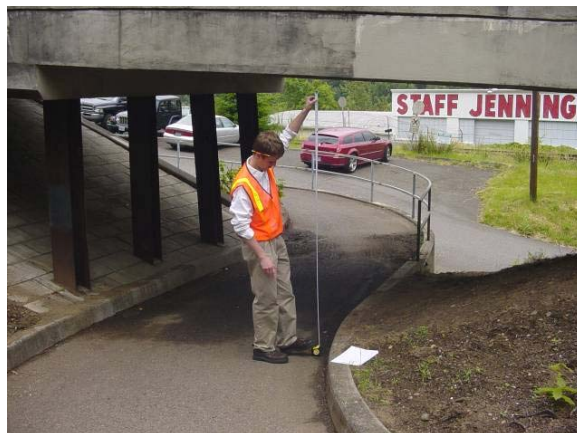
Figure 11: Vertical clearance of multi-use pathway beneath northbound bypass ramp is almost 3 feet lower than standard.
